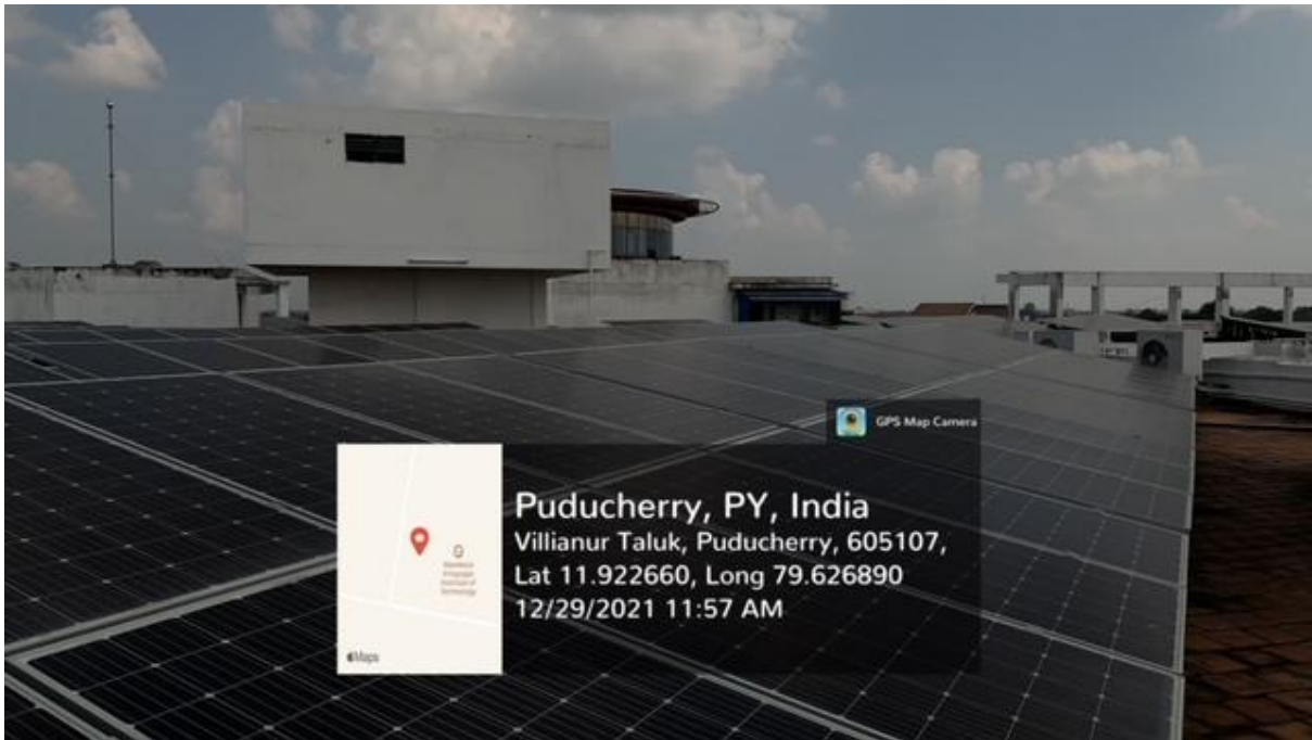
MVIT Solar PV PP for 311.71 kWp
